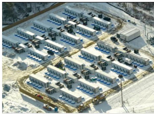
Figure 17 : Centrale de Stephentown
